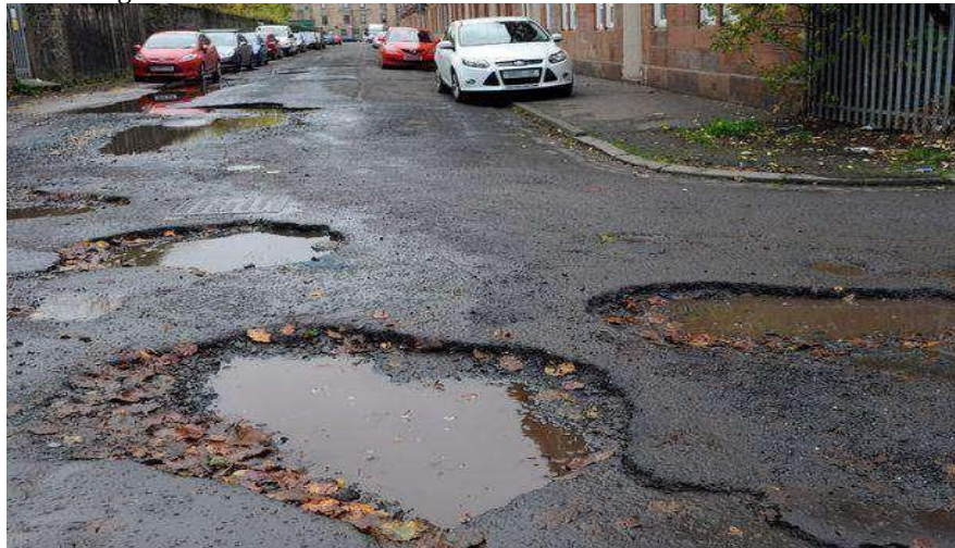
Fig:1.4 Potholes on roads
