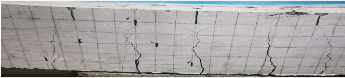
Figure Figure 18 : Crack pattern for control SCC beam
